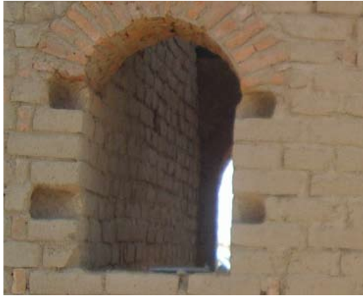
Pic 25. Four holes are made around the sides of the window hole
