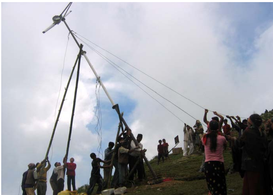
The community work together to erect a wind turbine in Phakhel village, Nepal
