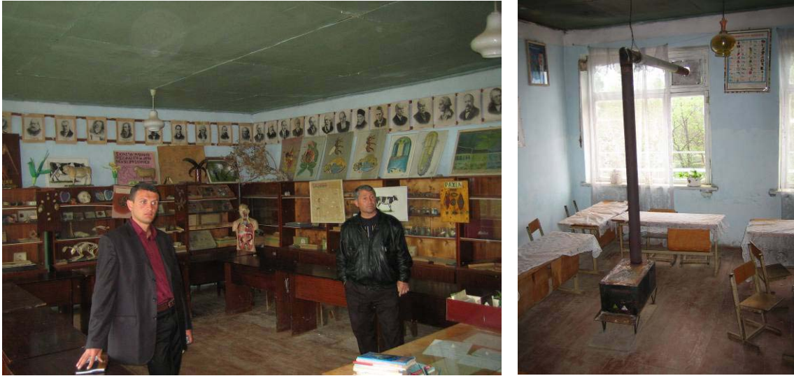
Figure 20 - Classroom in Yahdeli School showing ceiling (left) and wood burning stove (right)
