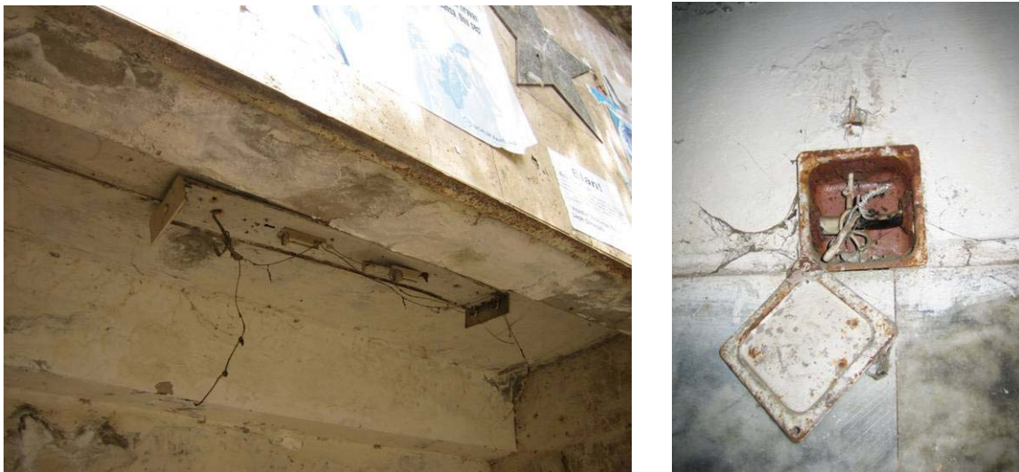
Figure 15 - One of few remaining original light fittings (left) typical wiring junction box (right)
