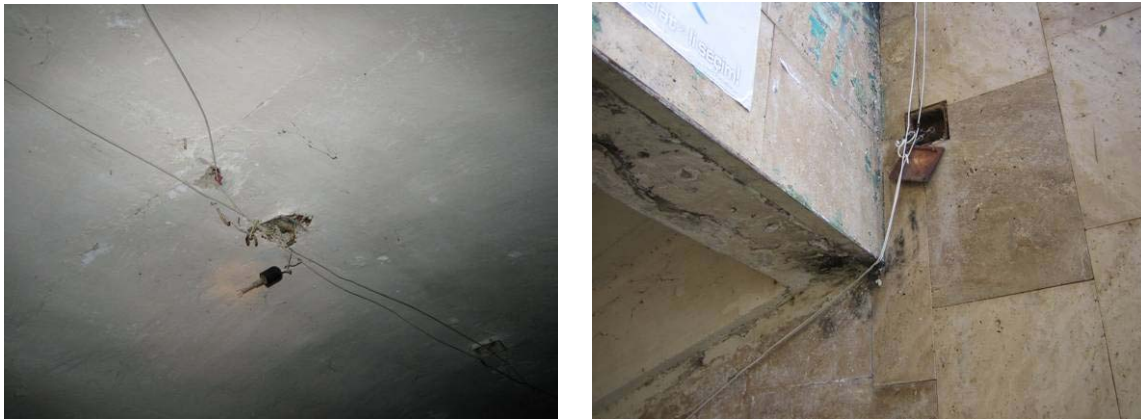
Figure 16 - Broken incandescent lightbulb and recent ceiling wiring (left) and recent wiring entering the underpass past soviet-era junction box (right)
