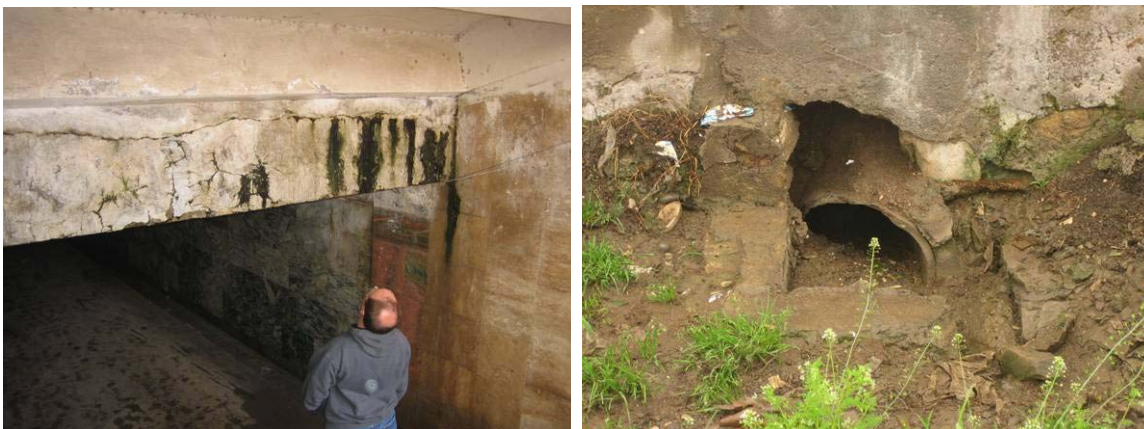
Figure 9 - Seepage inside southern end of underpass and blocked drain in railway siding above
