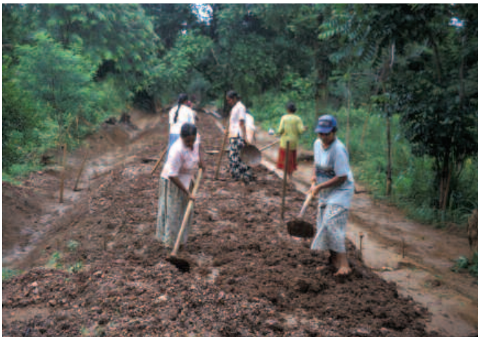
Women spreading a fine gravel as the surface layer of a community road which will be rolled later
