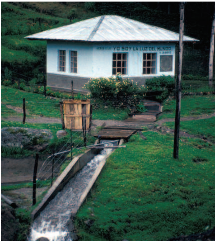
Micro hydro powerhouse in Peru showing water channel and transmission lines.
